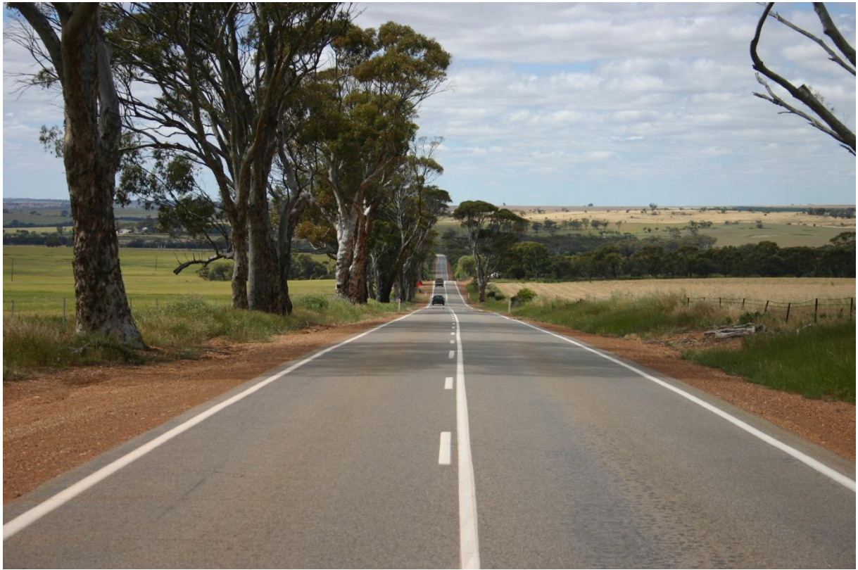
Photograph 2: Large eucalypts growing on west side of the road from SLK 18.2. Reconstructed section shown in Photograph 1 is located before the left hand bend in the distance. Washed out table drain commences before large tree on right hand side. Trees on the left range in age to in excess of 100 years.
