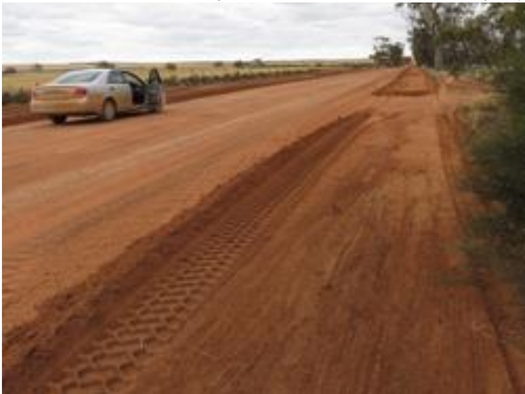
Koomberkine North Road: clearing fenceline to fenceline in areas not damaged by flooding
