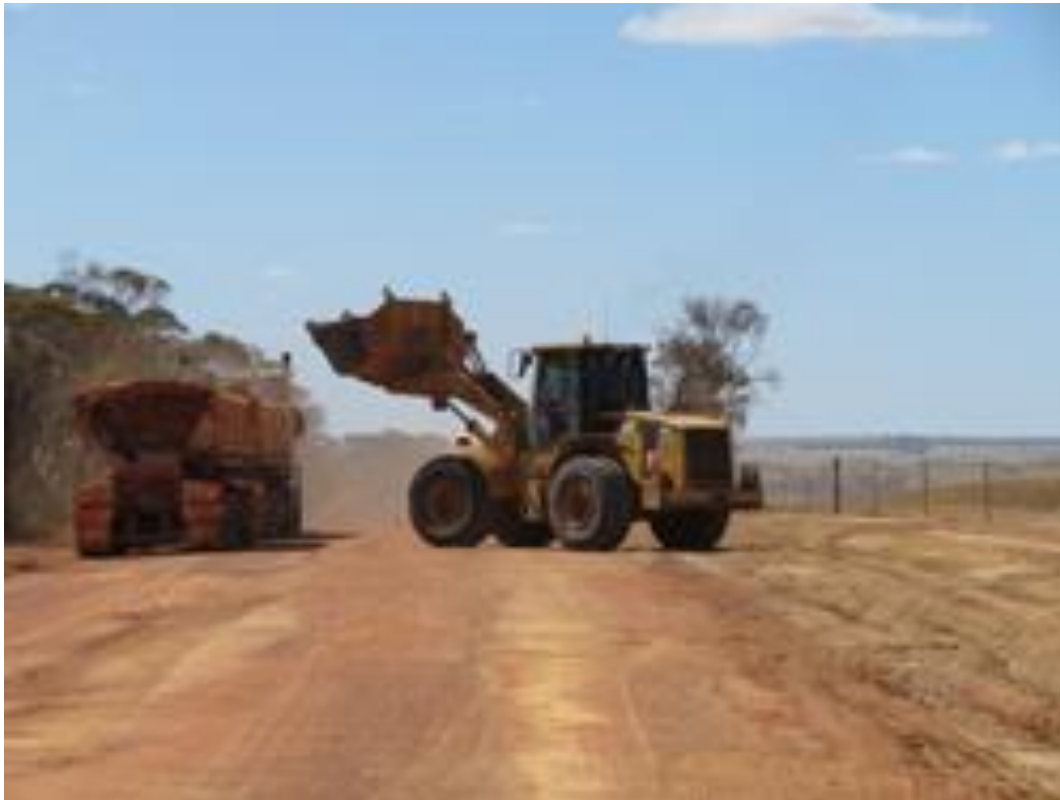
Clearing Uberin Road near Koombarkine Lake: massively cleared
