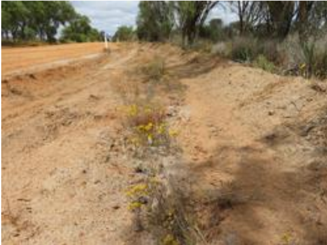
Uberin Road: destroying the wildflowers with too wide a drain/back slope
