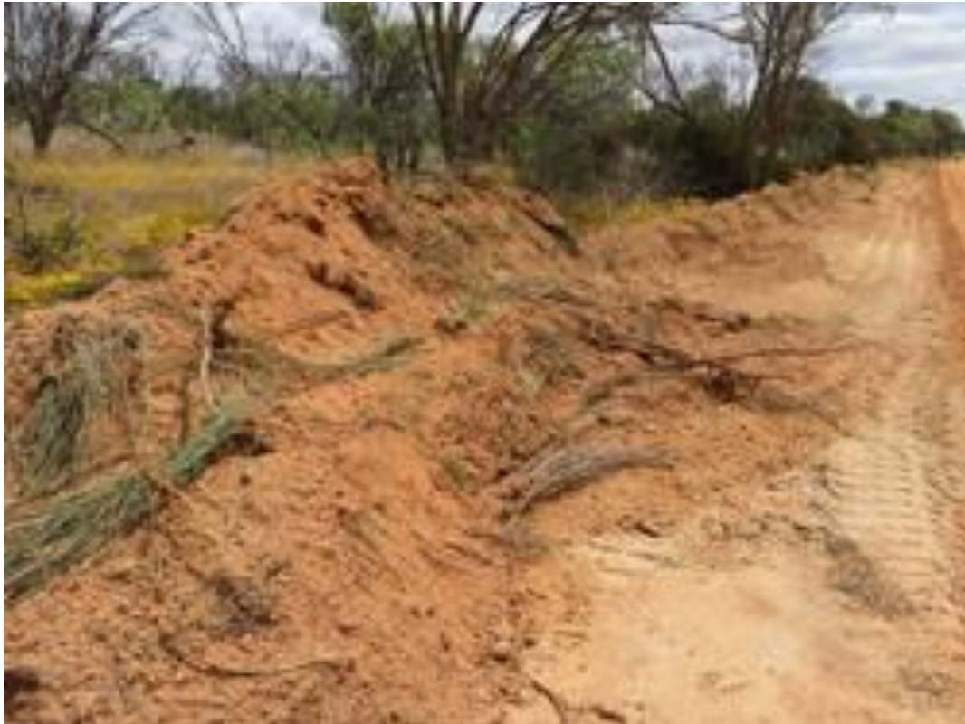
Uberin Road: excessive, destructive construction with too wide a drain/back slope
