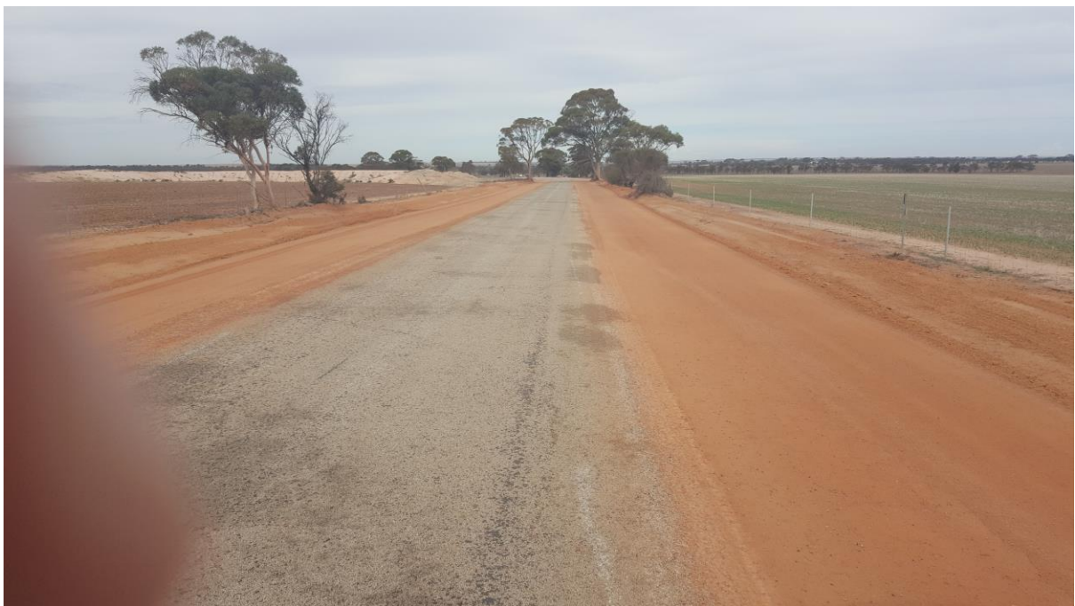
Photograph 2: Road widening carried out without a clearing permit which has removed all understorey.
