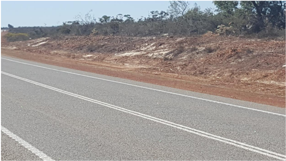
Photograph 1: Clearing outside the drainage requirements and lateral clearance requirements destabilising the backslope of the drain
